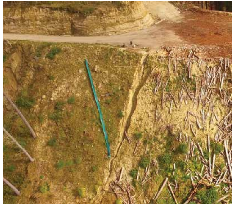
Inspecting erosion and water management in steep slope sites from a UAV. Source: Interpine
